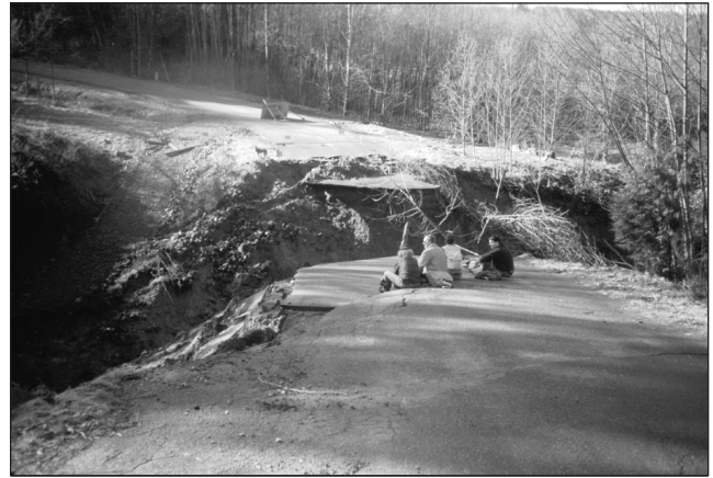
Road failure due to improperly installed culvert
